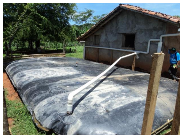
Figure 2: Rain Water Harvesting
